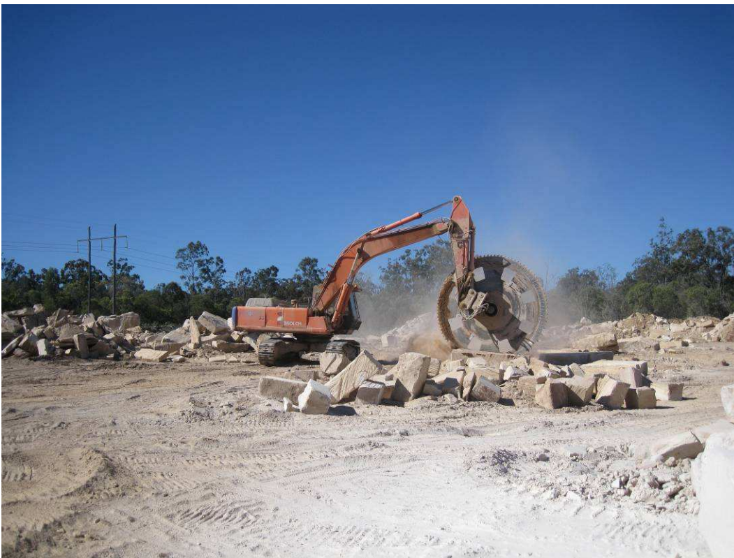
Photograph # 1; Airborne dust being generated from 350 LCH excavator saw attachment cutting sandstone.
